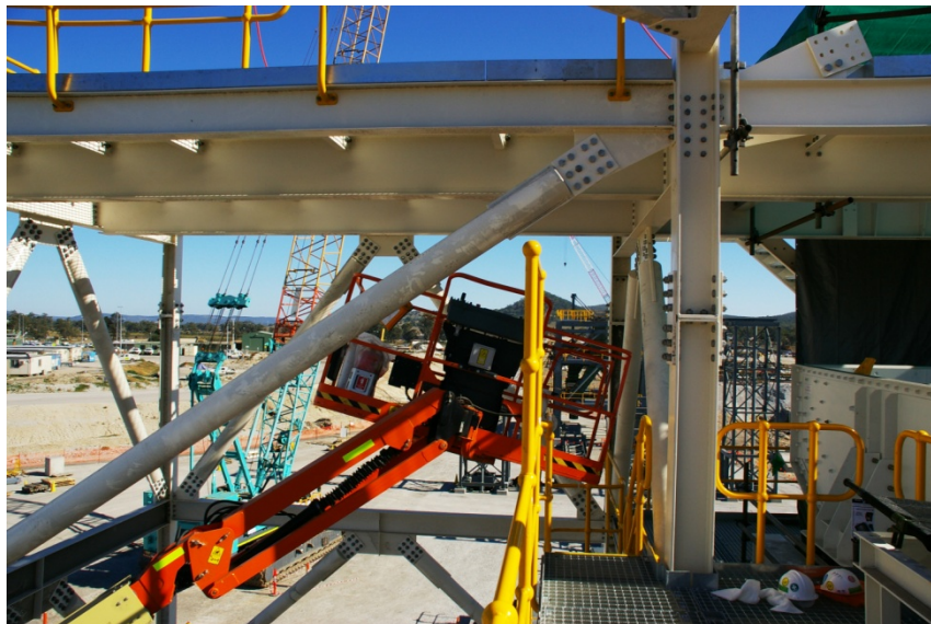
Position of MEWP basket (after recovery of worker) - Photograph by Investigation Unit
