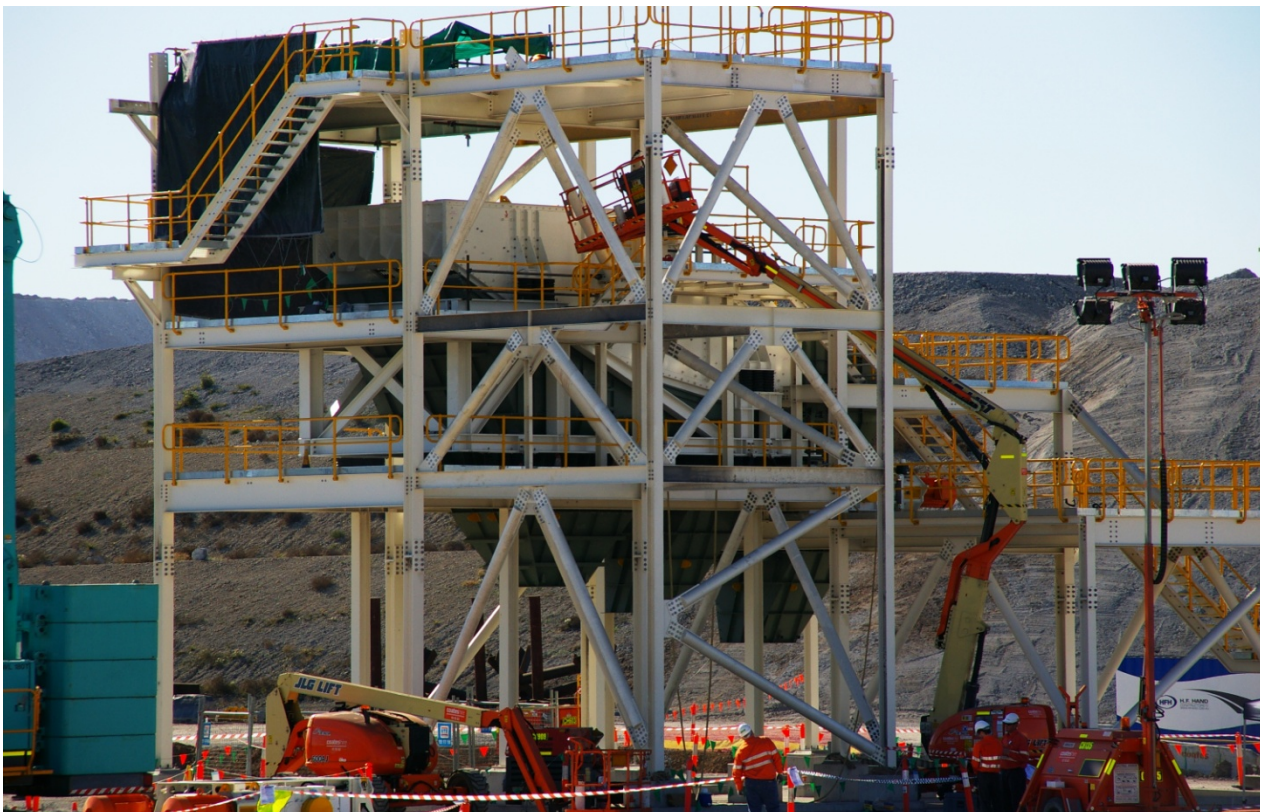
Steel structure with MEWP in approximate position (after recovery of worker) - Photograph by Investigation Unit
